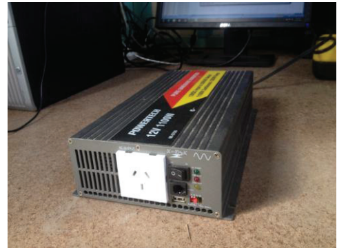
Figure 6: 1100W 12V inverter installed in energy system.
