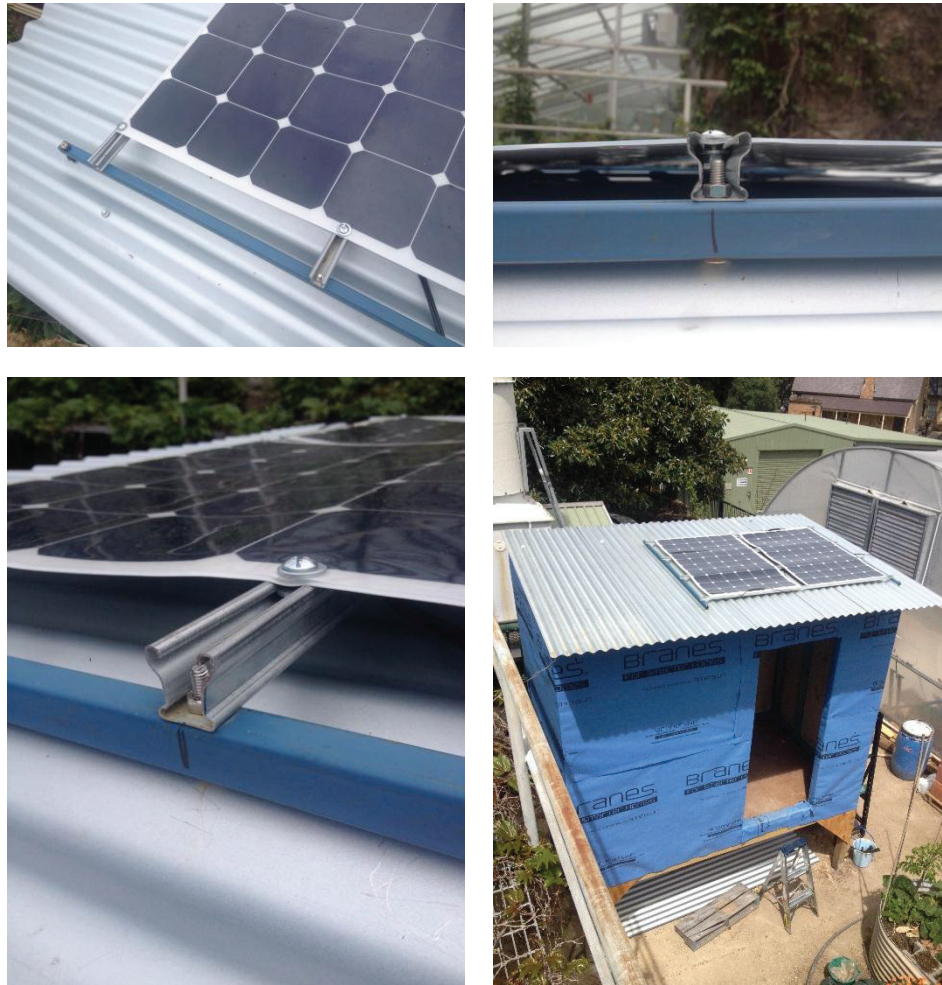
Figure 7: Mounting frame detail and mounting position of the solar panels on the roof.
